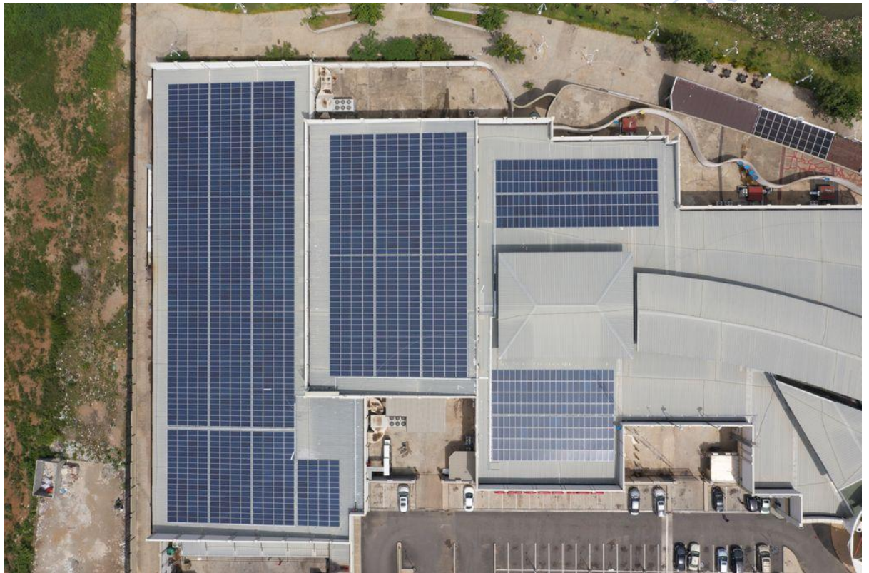
Figure 38; Solar panels covering the roof Source; Google
