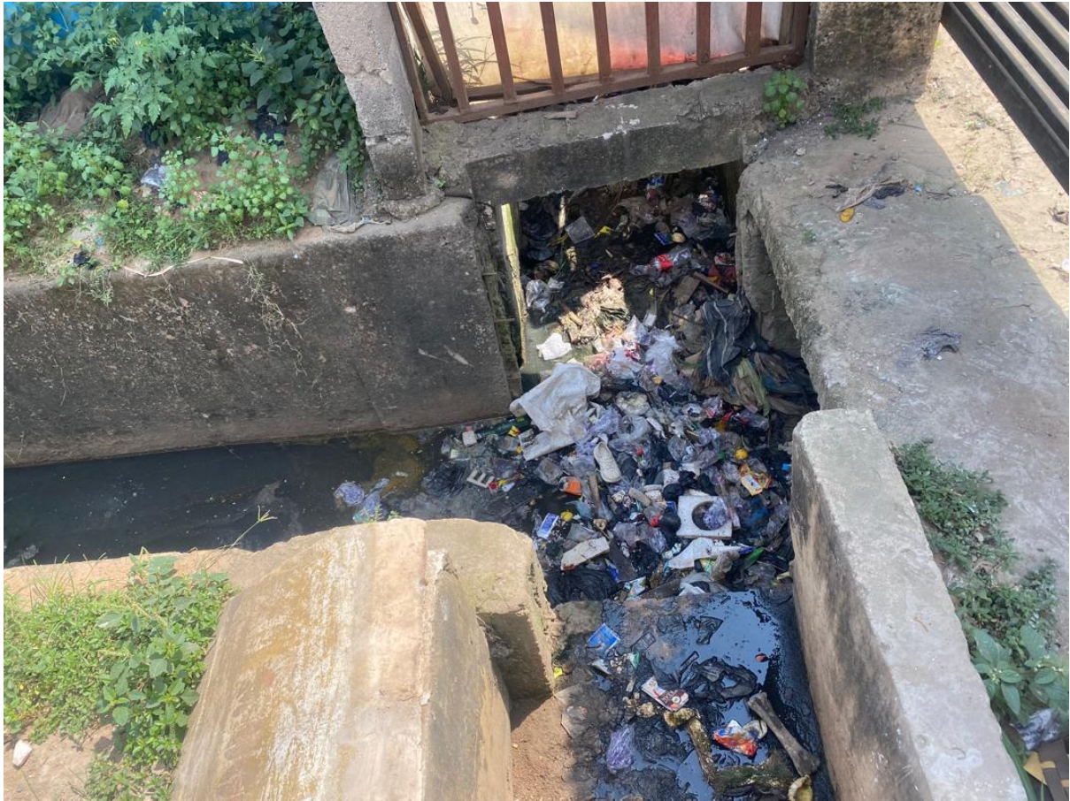
Plate 4.4: 16-year-old drainage constructed by the local government of Abule-Egba
