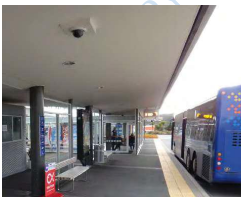
Figure 2.22: CCTV Camera Installed at the Loading-bay
