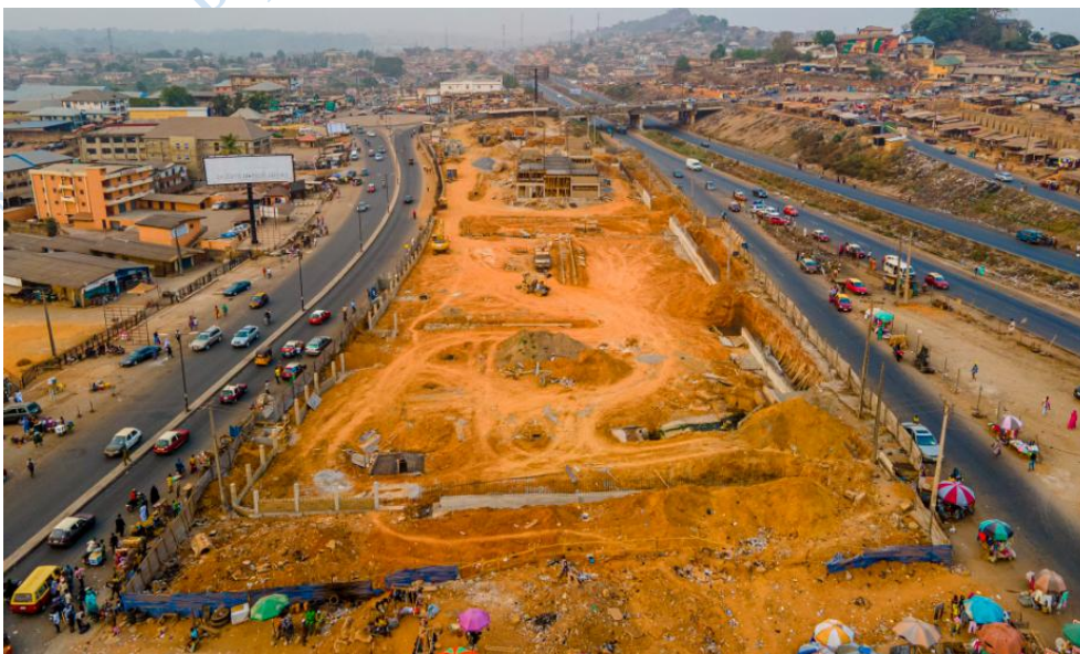
Figure 3.1: Site layout plan of the Modern Bus Terminal at Ojoo in Ibadan.
