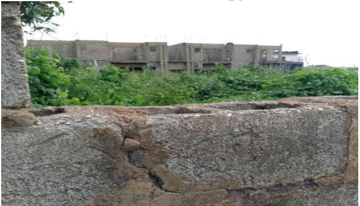
Plate 4.10: Abandoned Residential Buildings at Obasanjo Hilltop Housing Estate,
