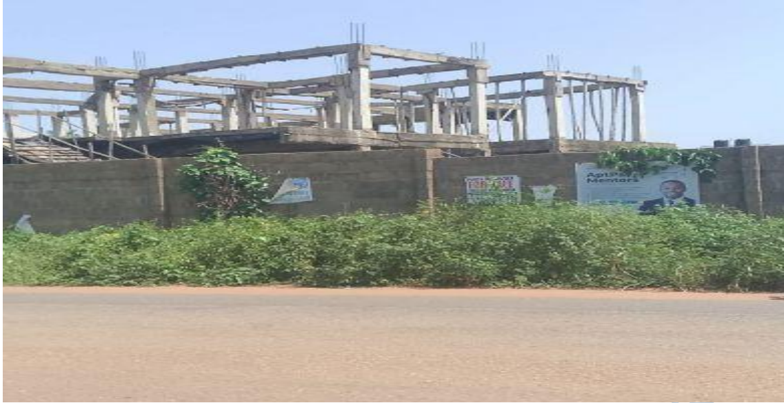
Plate 4.7: Abandoned Residential Buildings at Obasanjo Hilltop Housing Estate, Abeokuta
