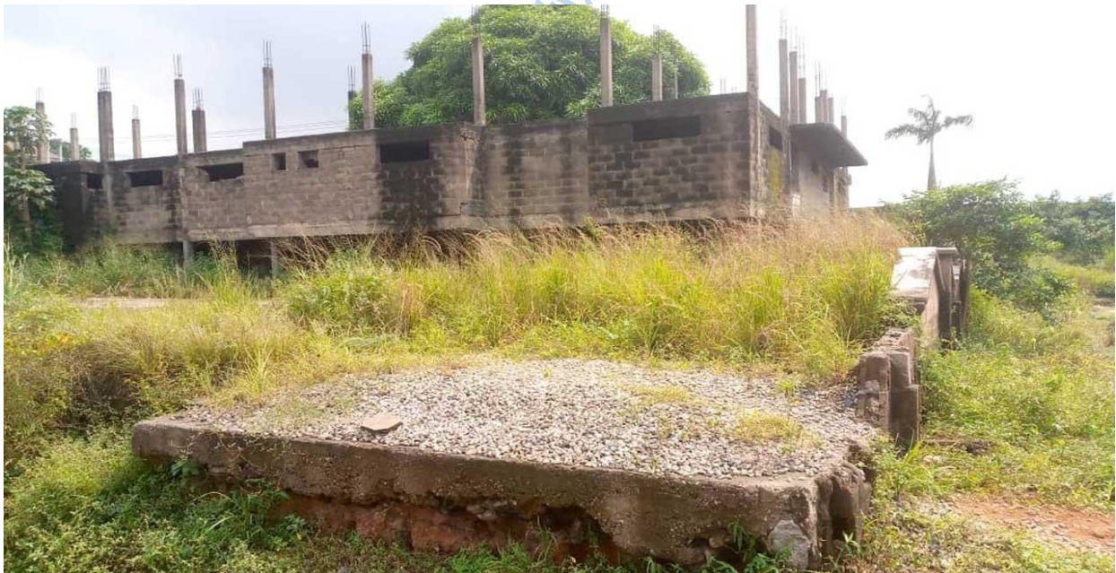
Plate 4.28: Abandoned Residential Buildings at Ibara Housing Estate, Abeokuta Ogun State. Source: Field Survey, January, 2024
