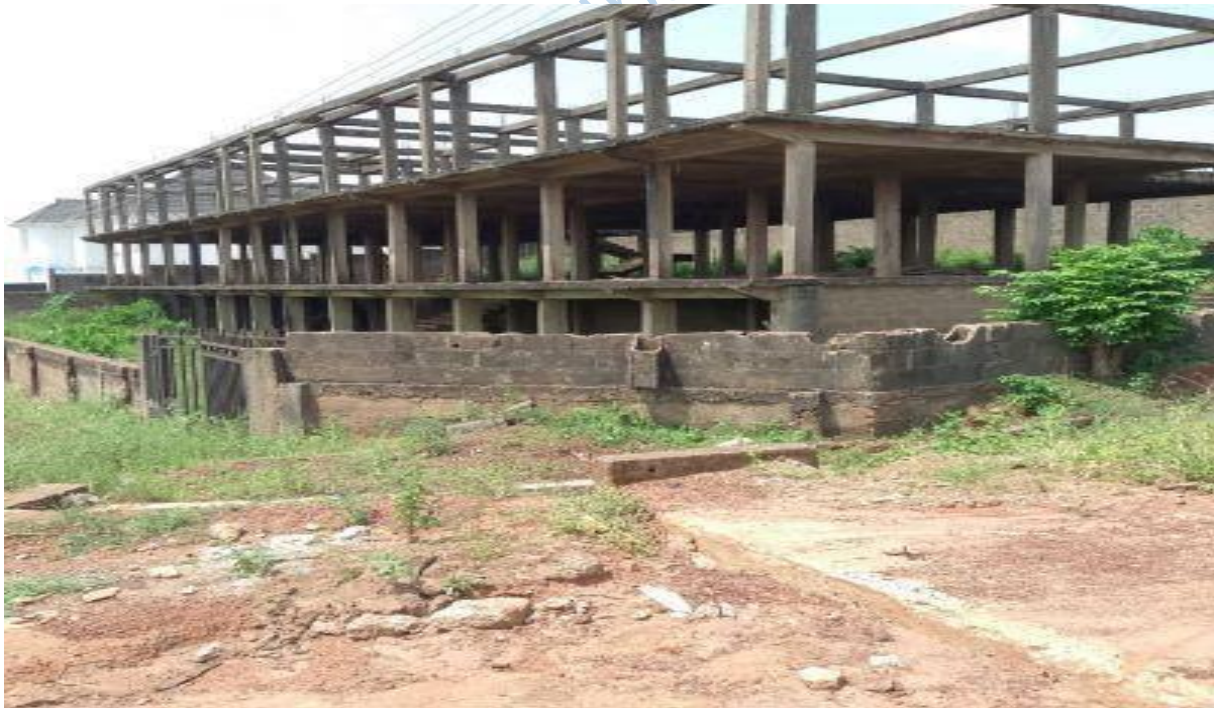
Plate 4.14: Abandoned Residential Buildings at Obasanjo Hilltop Housing Estate, Abeokuta Ogun State.
