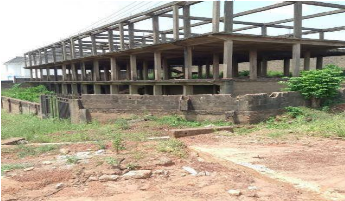
Plate 4.14: Abandoned Residential Buildings at Obasanjo Hilltop Housing Estate, Abeokuta. Source: Field Survey, October, 2024
