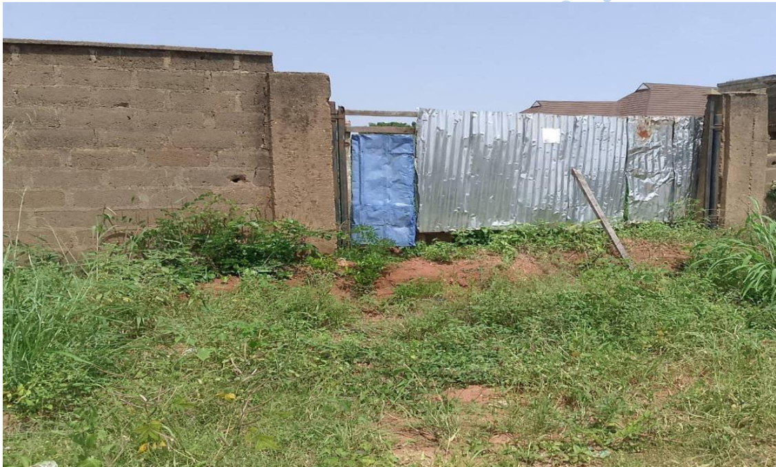
Plate 4.4: Abandoned Residential Buildings at Laderin Housing Estate, Abeokuta.
