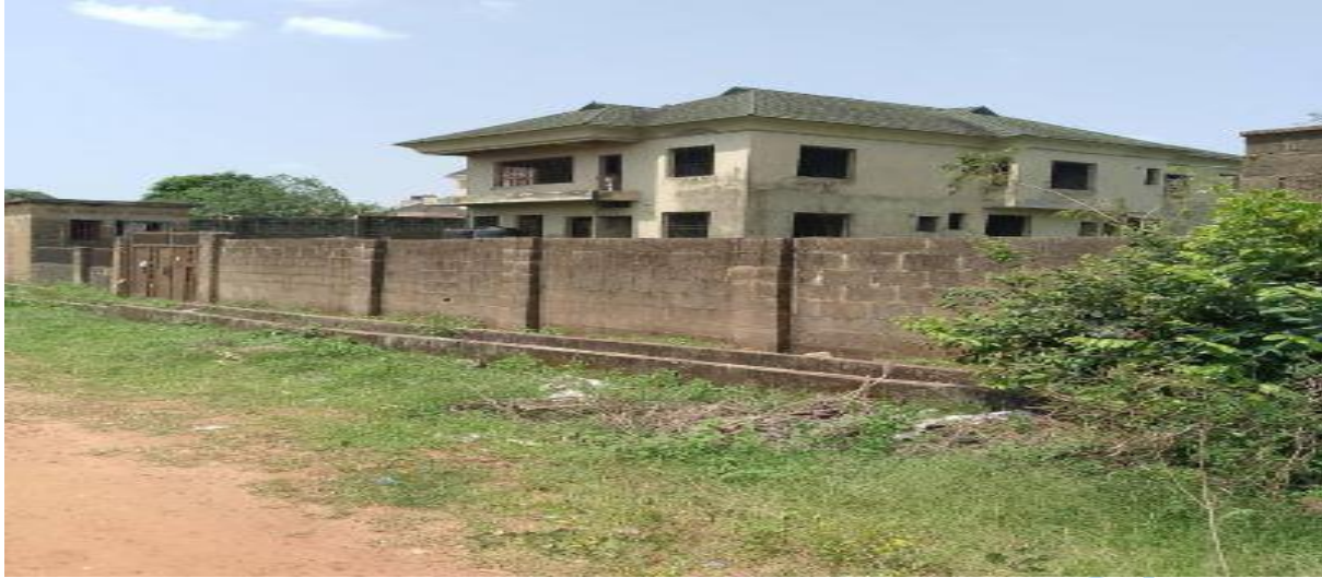
Plate 4.13: Abandoned Residential Buildings at Obasanjo Hilltop Housing Estate, Abeokuta. Source: Field Survey, October, 2024
