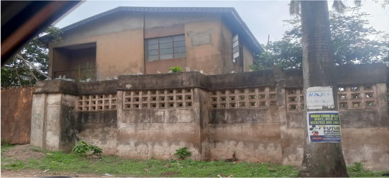
Plate 4.17: Abandoned Residential Buildings at Obasanjo Hilltop Housing Estate, Abeokuta Ogun State.
