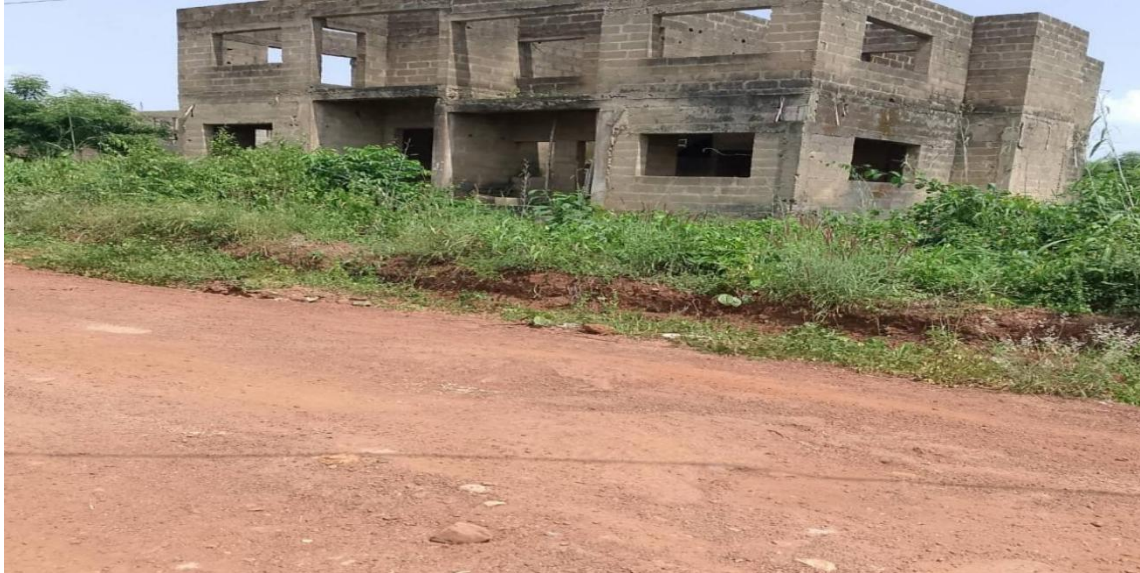
Plate 4.1: Abandoned Uncompleted Residential Buildings at Laderin Housing Estate, Abeokuta
