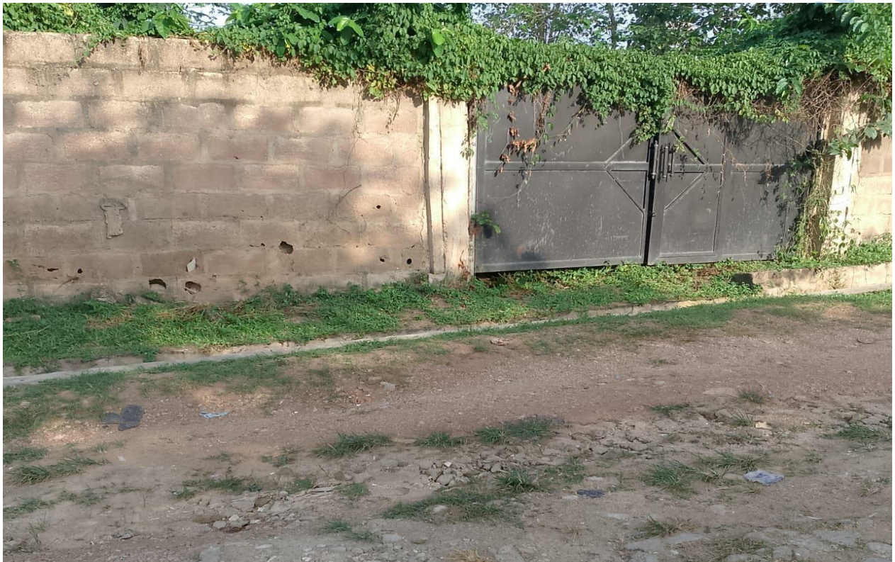
Plate 4.29: Abandoned Residential Buildings at Ibara Housing Estate, Abeokuta Ogun State. Source: Field Survey, January, 2024
