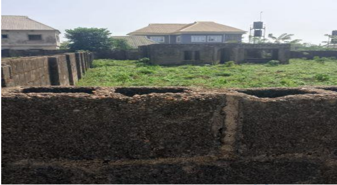
Plate 4.11: Abandoned Residential Buildings at Obasanjo Hilltop Housing Estate, Abeokuta. Source: Field Survey, October, 2024
