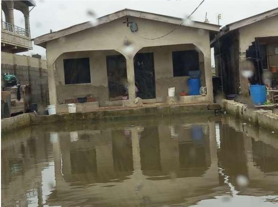
Figure 4.15: Water penetration damage to building in the Ajegunle area. Source: Researcher's Field Survey, (2023)
