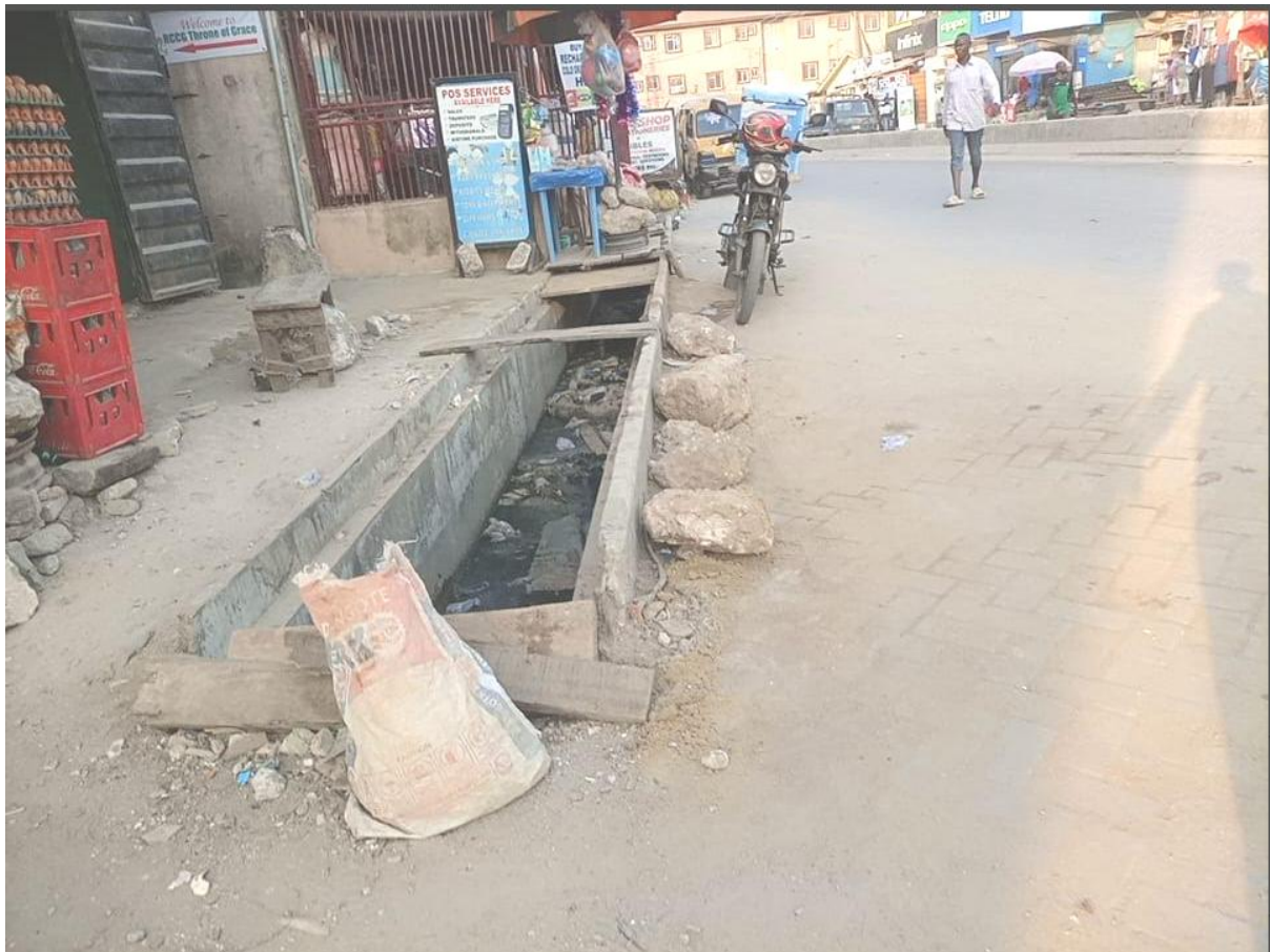
Picture of the advanced or more organized area in the slum settlements with an unhealth drainage system
