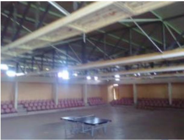
Figure 57: Interior view of the multipurpose court, O.A.U Sports Hall
