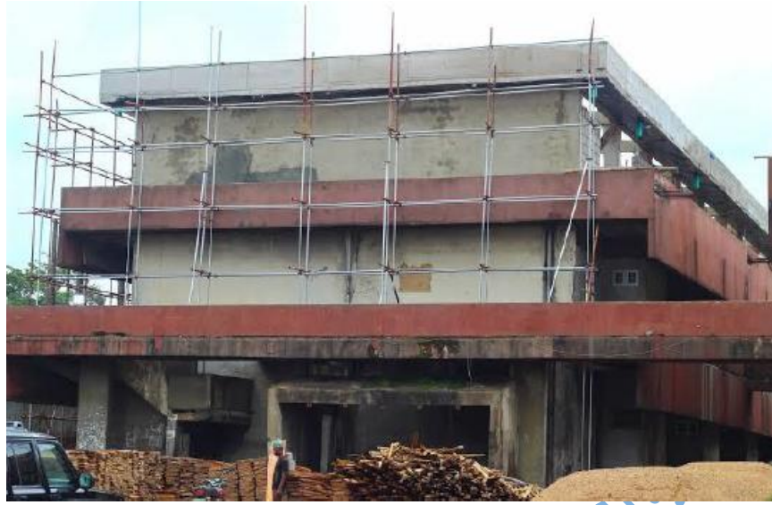
Plate 4.4: Image showing side view of abandoned Agbowo Mall Source: Researcher's Archive, 2023
