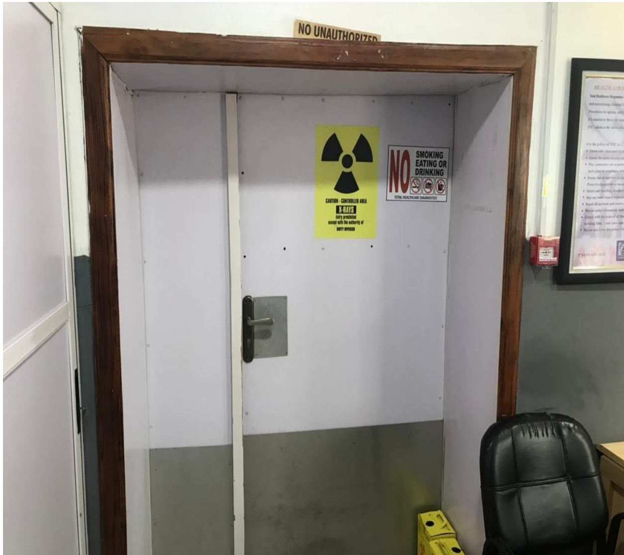
Figure 3.20: picture of door with well lead lining in facility E.
