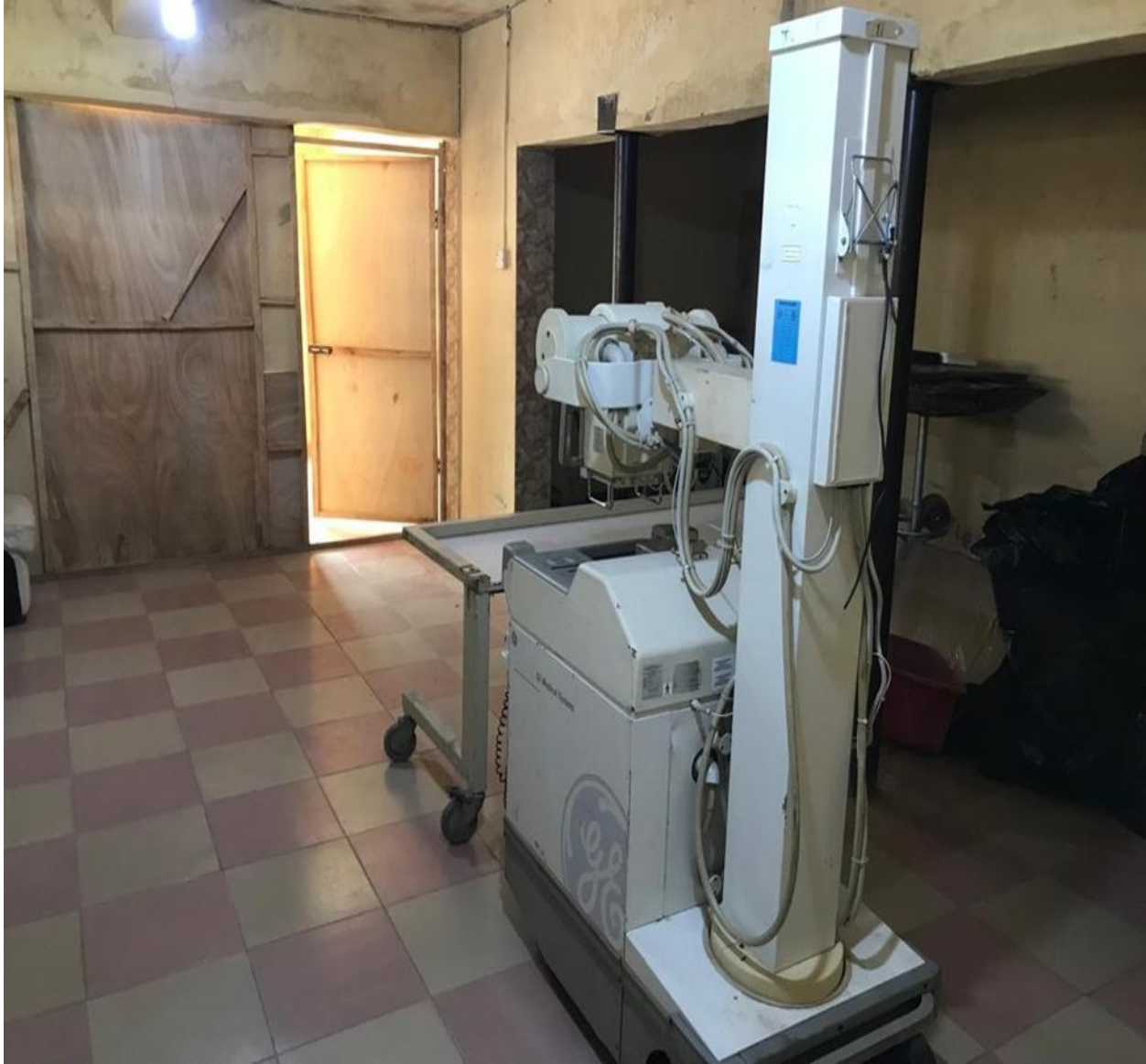
Figure 3.11: Picture from Centre G, showing the wooden door without any lead lining
