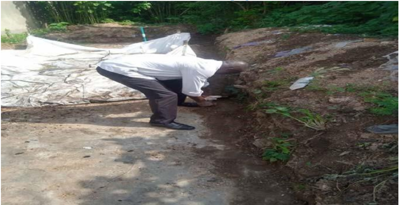
Plate 4.2: Cleaning of sanitary landfill prototype for easy passage of water by the researcher
