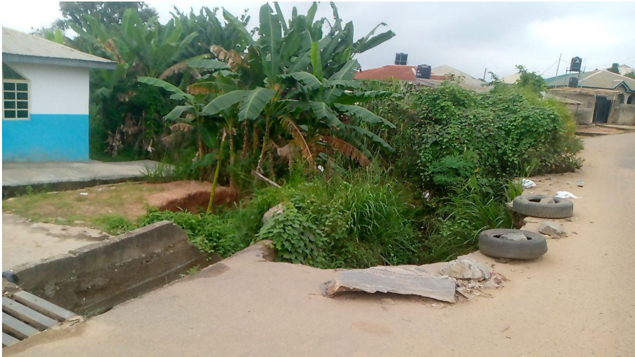
Figure 4.67. Land Degradation Effect Part of Road and on Building Foundation Due to Flooding Source: Fieldwork 2023
