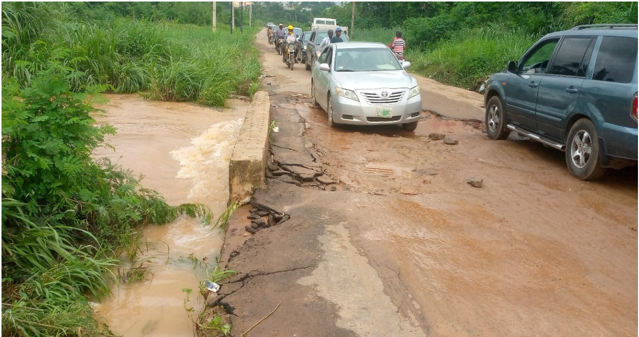
Figure 4.63 Increase in Water level and annual flooding effects on Road Infrastructure
