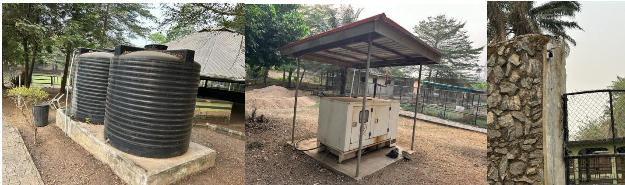
Plate. 4.6: Service (Water Station, Generating Plant, CCTV Camera) (Source: U.I Zoological Garden, 2024)
