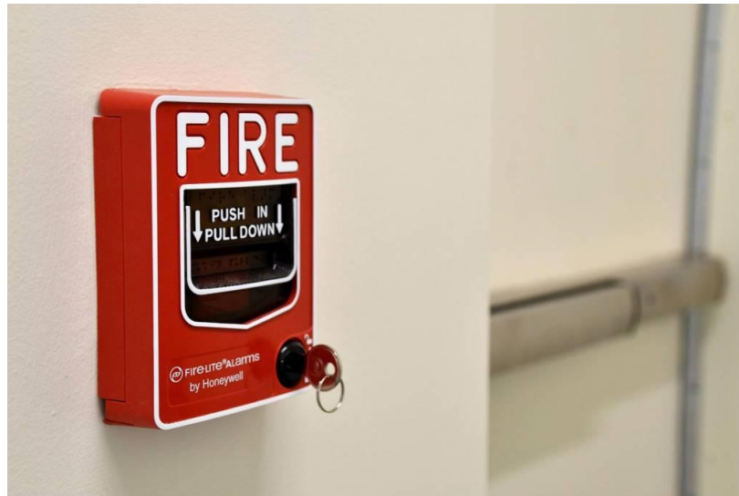
Figure 3 - Fire alarm. (Source: Google Imagery, 2022)
