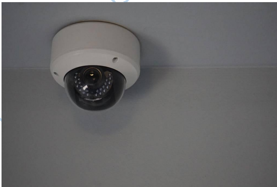
Figure 2 - Security camera. (Source: Google Imagery, 2022)
