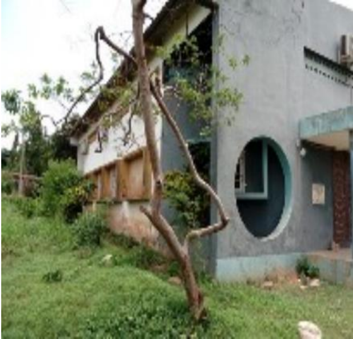
Figure.3.19. Main Conference Hall: Rotary Club House – Ibadan Side Elevations (Source: Author’s Field Work)
