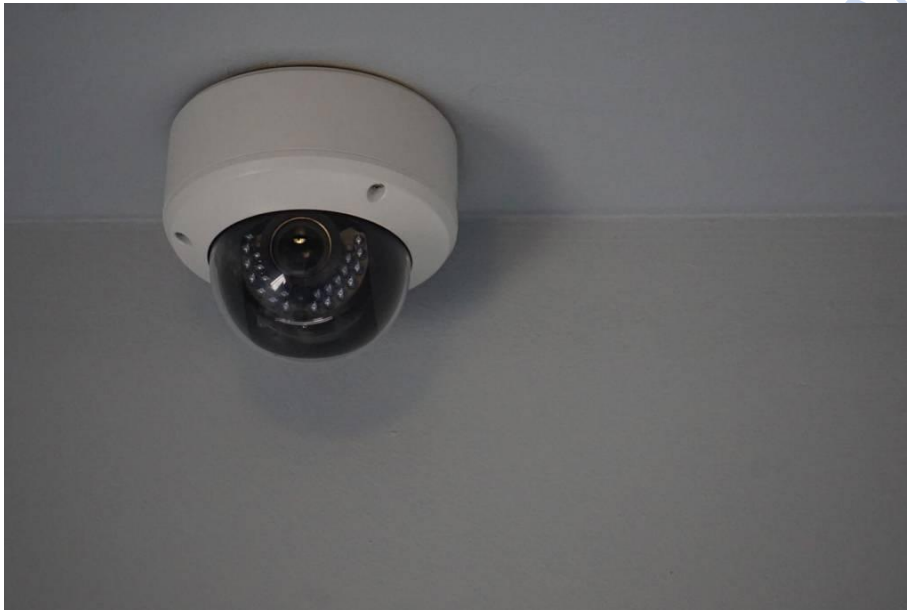
Figure 2.2: Security camera Source: Author's field survey
