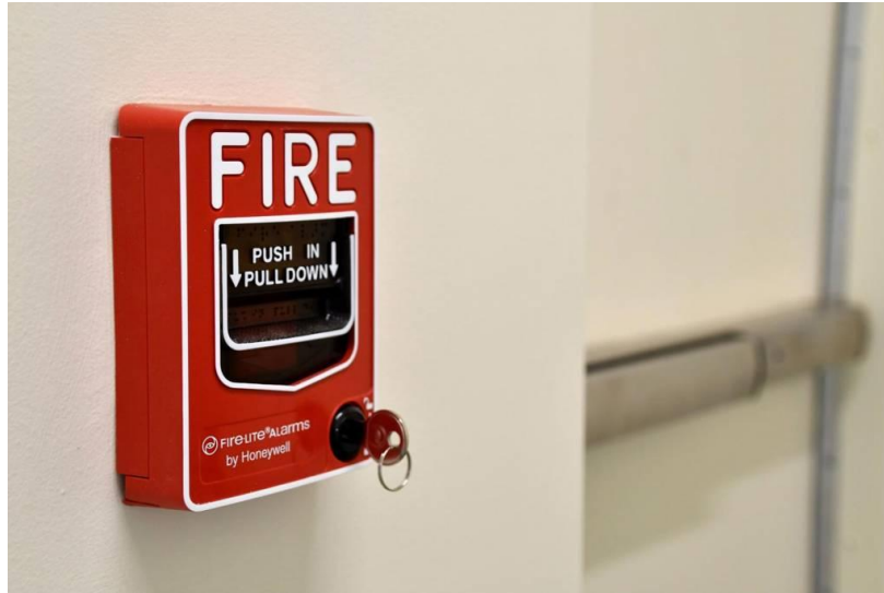
Figure 2.3: Fire alarm Source: Google Imagery, 2022
